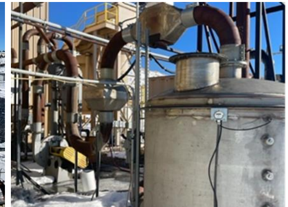
Deep Bed Scrubber
