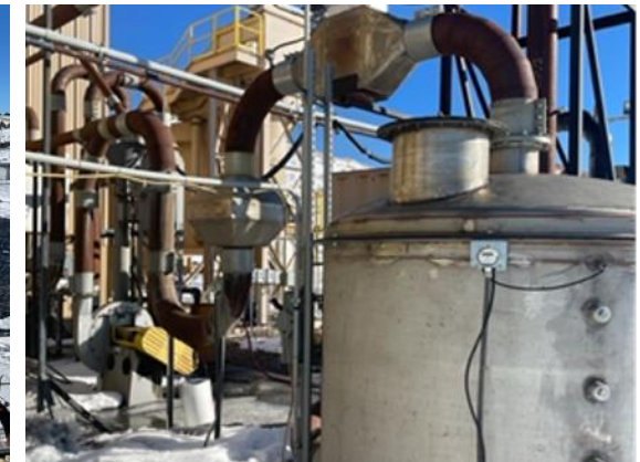
Deep Bed Scrubber
