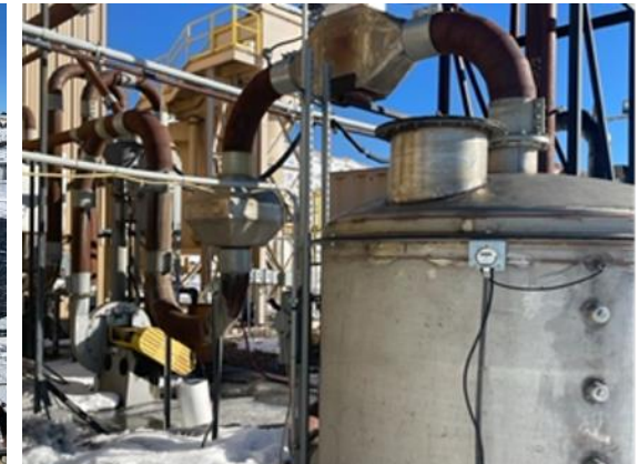
Deep Bed Scrubber
